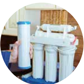
Reverse Osmosis System (found under the sink)
